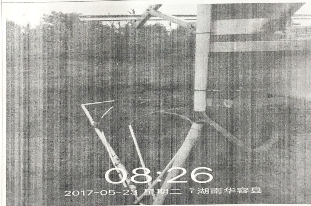
汇流箱引出线应穿波纹管保护
