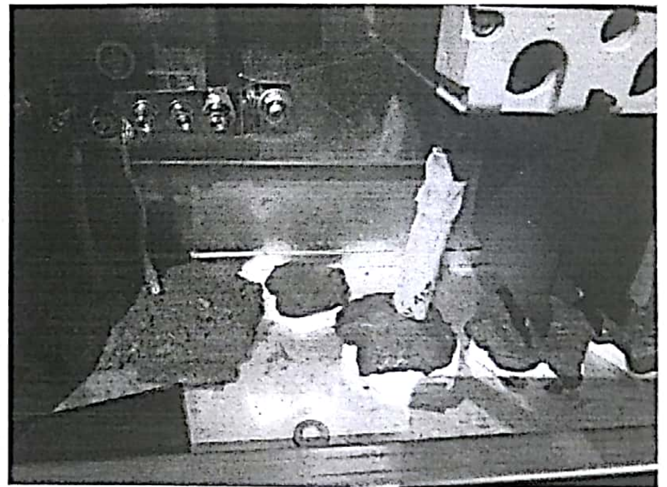
洞口防火泥封堵观感差、不规范
