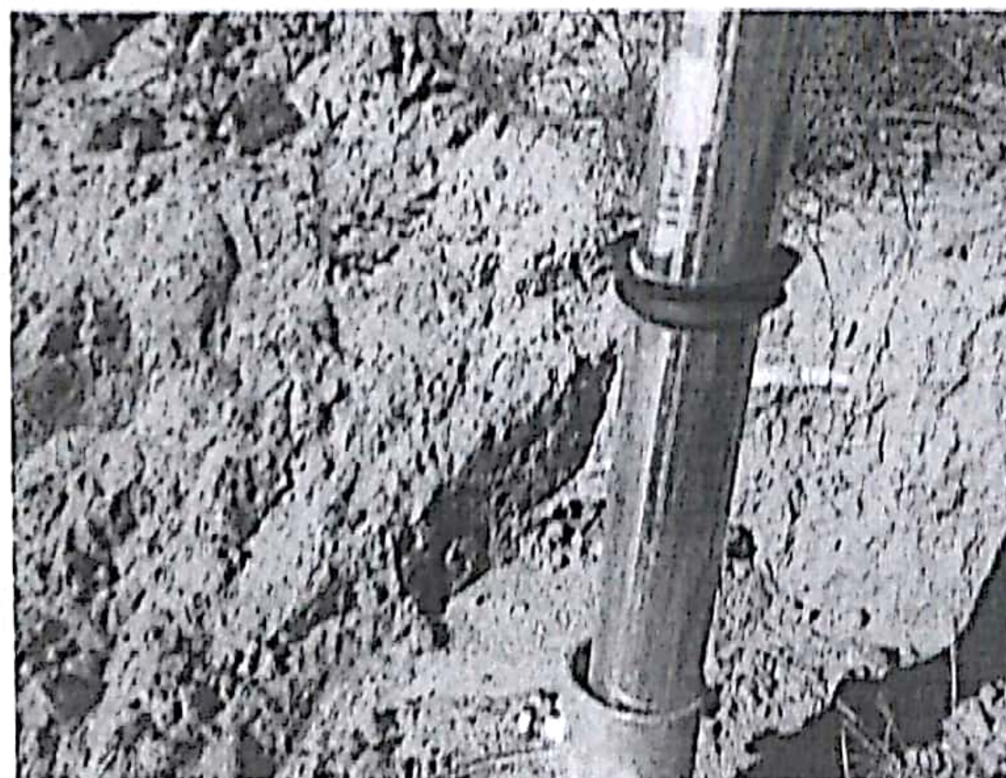
支架防水皮套翻口朝向错误
