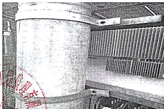
汇流箱支架、螺栓锈蚀
