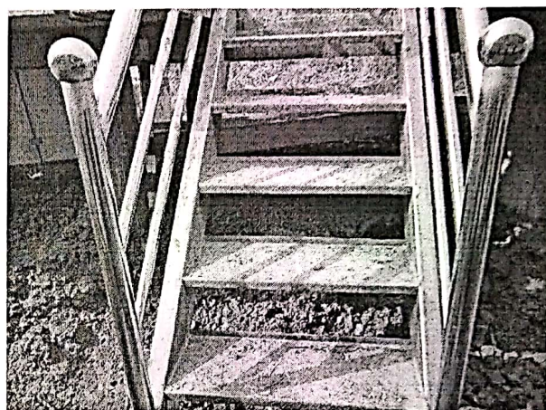
箱逆变平台爬梯除锈防腐未做
