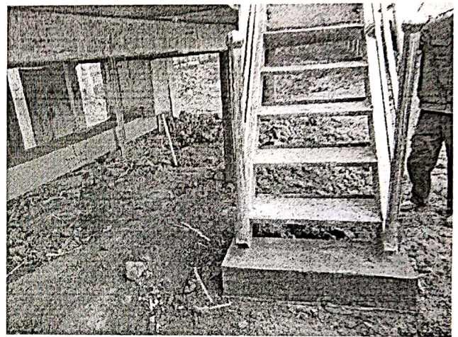
箱逆变平台爬梯除锈防腐未做
