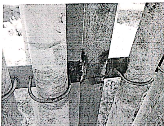
汇流箱支架焊接未防腐
