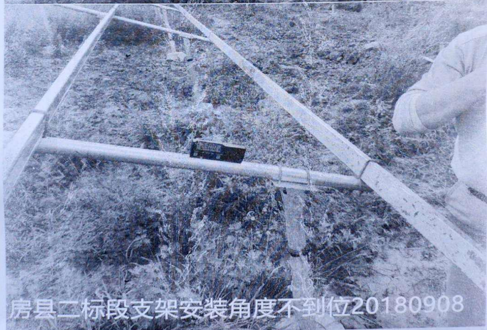
房县二标段支架安装角度不到位20180908
