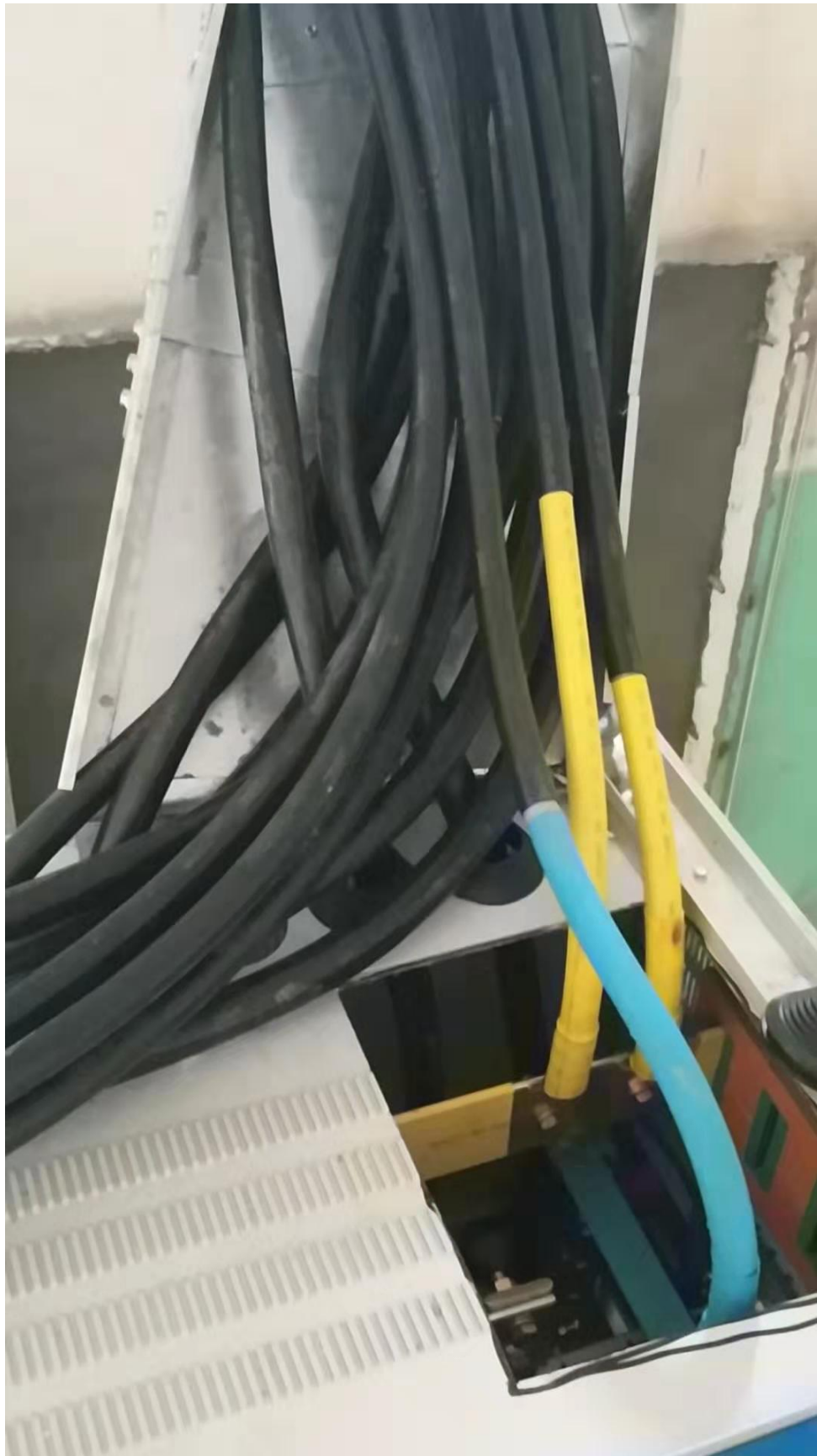
附图十：进配电室电缆杂乱
