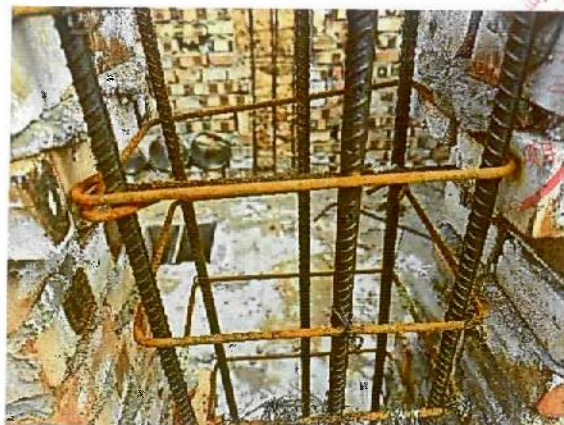
构造柱钢筋未满扎
