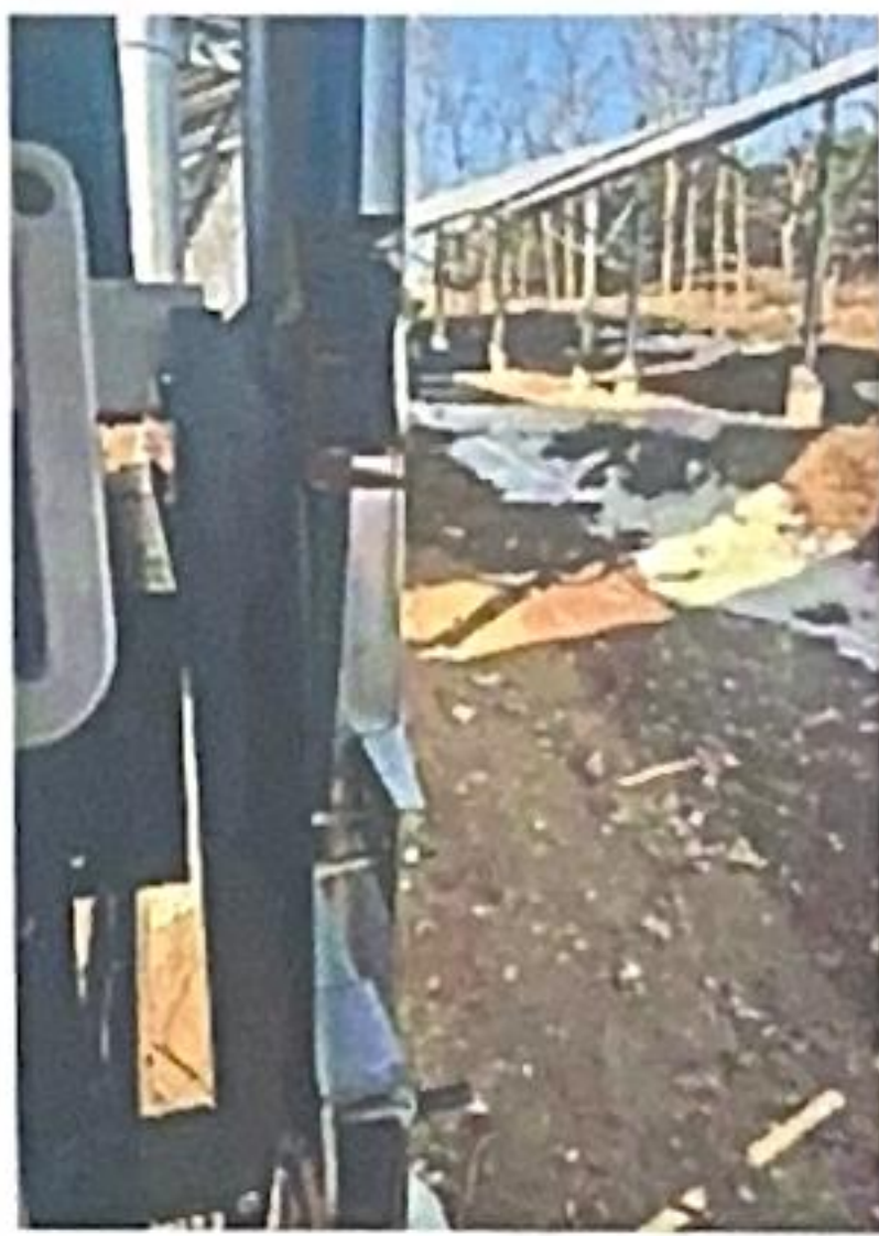
2、逆变器支架多处生锈
