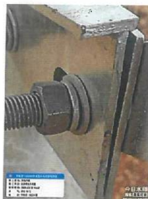
2、拉筋螺栓未紧固
