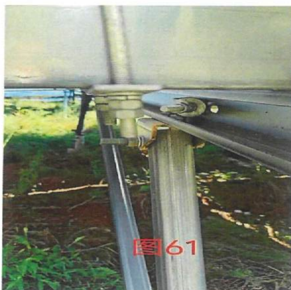
右侧组压块未安装垫片已整改
