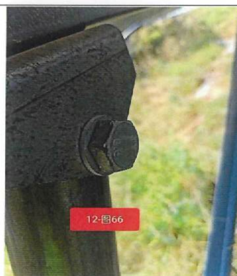
螺栓生锈已整改
