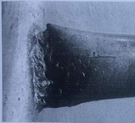
爬梯踏步焊接不牢固
