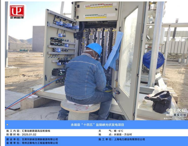
汇集站高压开关柜接线
