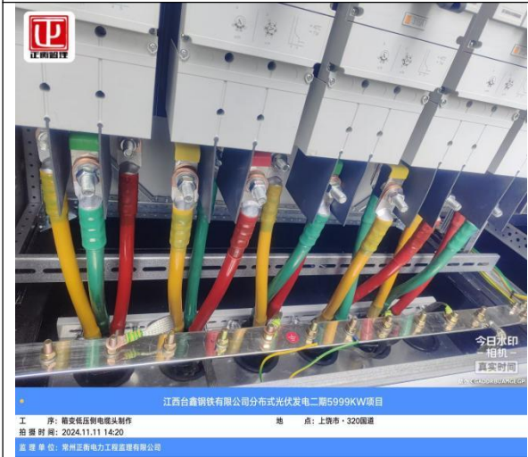
箱变低压侧接线
