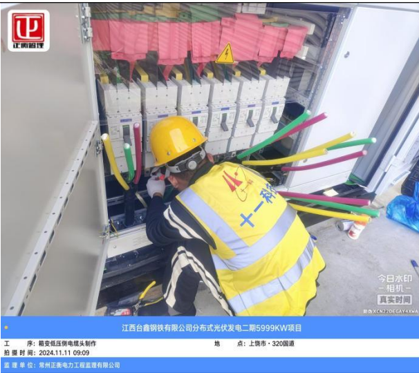
箱变低压侧接线
