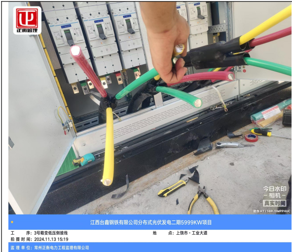
3#箱变低压接线
