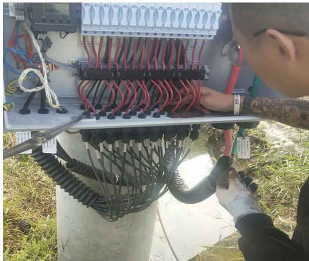
14#汇流箱防火 封堵
