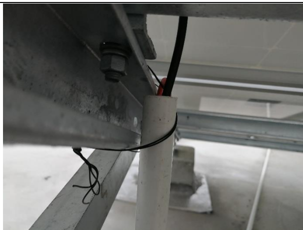
组件下接线管口未封堵
